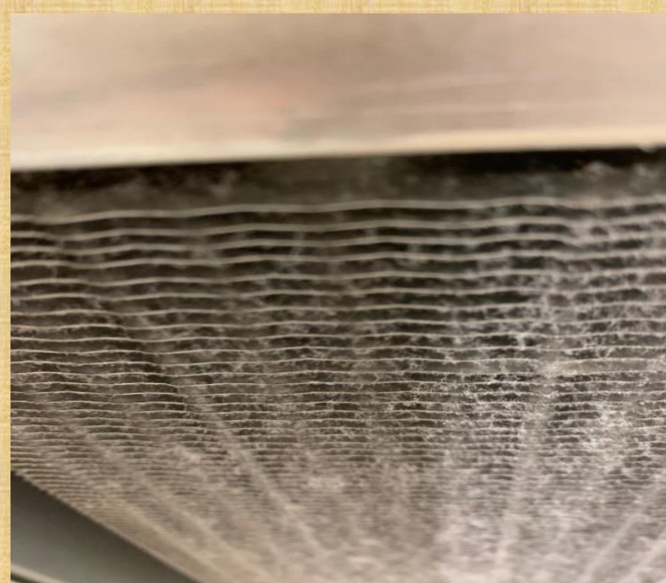
CHILLED BEAM IN BEDROOM CEILING
